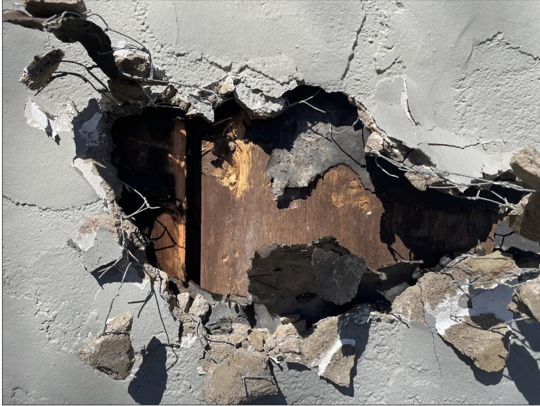
Photograph 16. Photograph of original siding exposed beneath stucco, facing north on south elevation.
