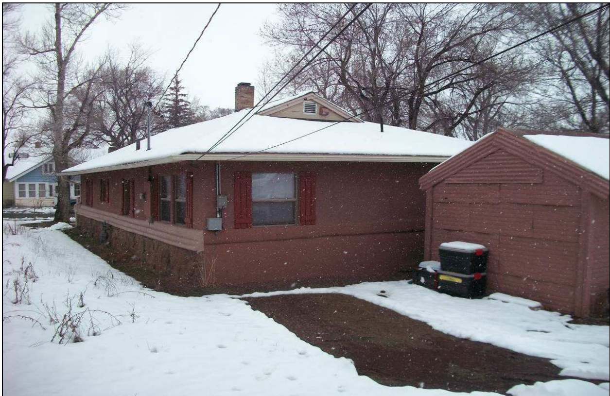
Figure 2. Gable roof, Dutch gable roof at south end, and central chimney, facing north-northeast.
