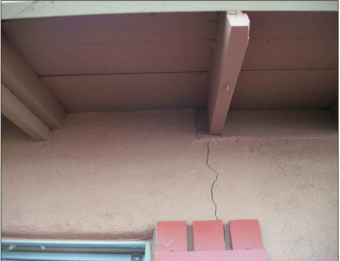
Figure 6. Seam connecting original structure (right) and addition (left) along east wall, facing west.
