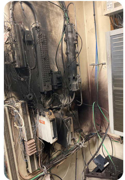
Damaged power supply boxes at Wildcat Hill WRP.
