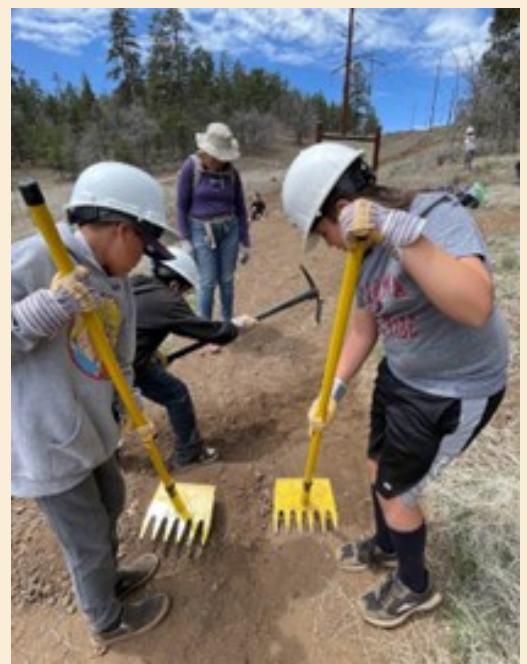
Right: Students use their tools to dig out a drainage canal and tamp down the berm.
