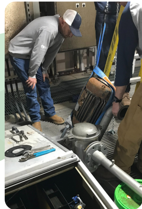
Staff inspect equipment impacted by high flows at Wildcat Hill Water Reclamation Plant
