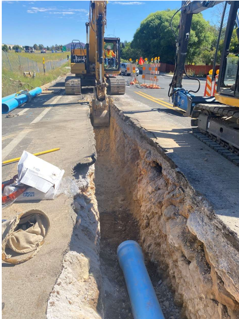
Installation of the new 12” PVC water transmission main, looking west on Soliere Ave.
