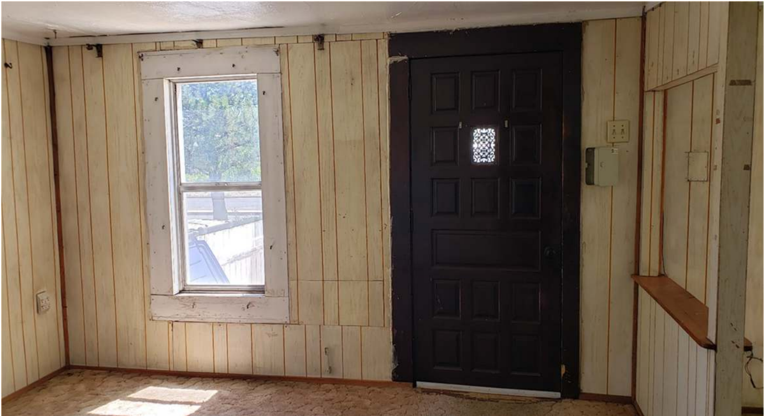
Photos 23–24. 609 S Lone Tree Rd E/front door exterior (top) and front door/NE corner room facing E (bottom).
