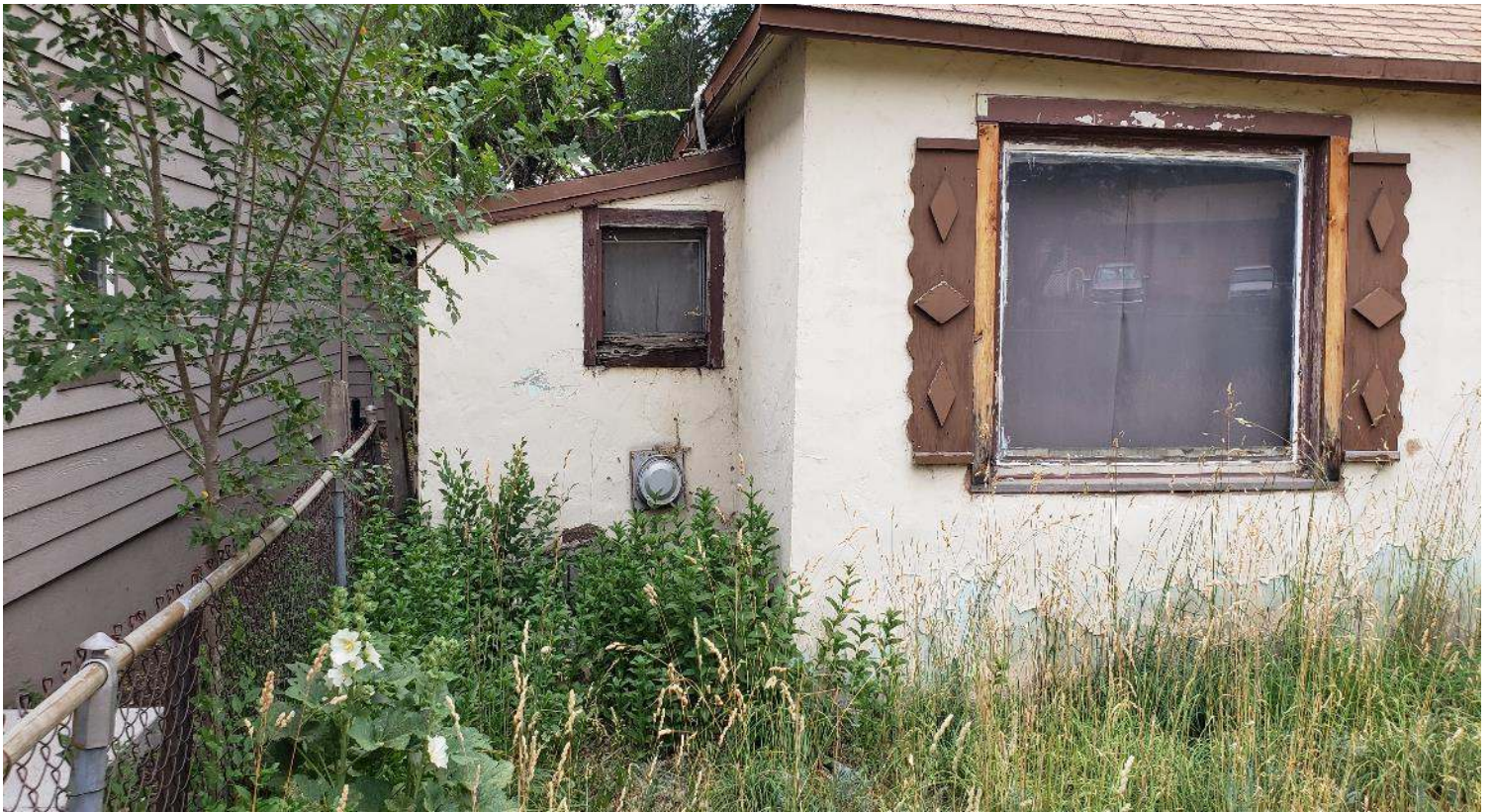
Photos 17–18. 617 W Tombstone Ave W façade N half windows (top) and aluminum and fixed windows on the front/N façade (bottom, bathroom to left and enclosed veranda room to right).
