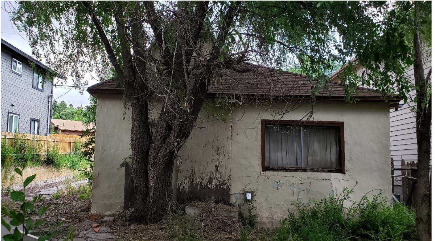
Photos 7–8. 617 W Tombstone Ave front/N façade facing SSW (top) and rear/S façade facing N (bottom).
