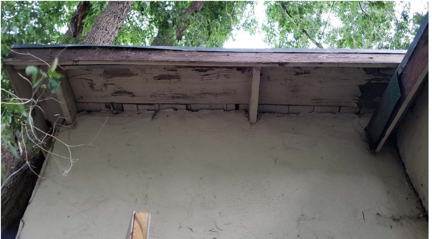
Photos 61–62. 617 W Tombstone workshop screened window in S façade (top) and eave over building's S half N façade entry (at NE corner of S half) facing up/S (bottom).
