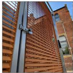
1. Access door - Steel
