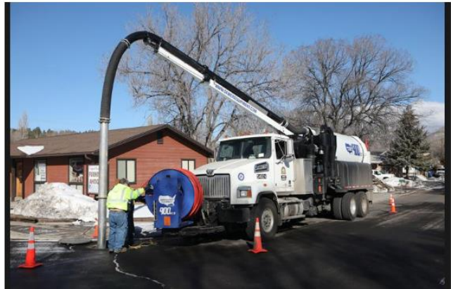
City of Flagstaff stormwater maintenance worker Paul Wolf feeds a pressure washer into a manhole to wash out accumulated sediment nearby blocking the stormwater tunnels under a street in Sunnyside in this 2023 photo. Jillie Slocum, Arizona Daily Sun
