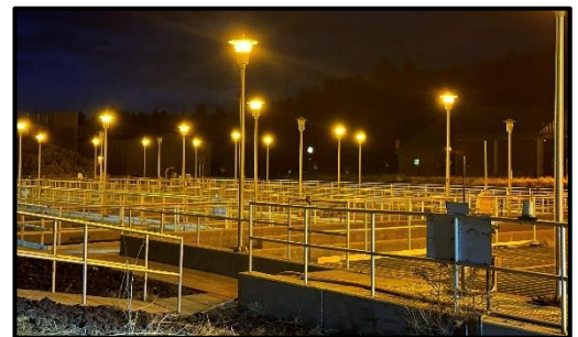
Photo: The Wildcat Hill Water Reclamation Plant at night, with new LED lights.
