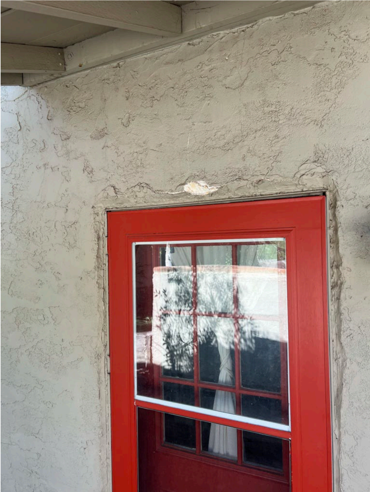
Photos of Current Conditions – 823 W. Aspen Ave. August 2024
