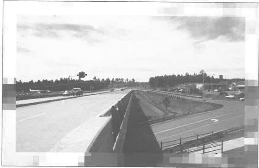
The Interstate 17/Interstate 40 interchange on the south side of Flagstaff is currently undergoing a major expansion to handle increased traffic more efficiently. The increased demand for such development underscores the importance of implementing a region-wide plan for determining the course of future development and controlling its pace.
