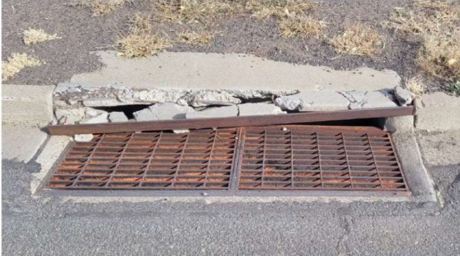
Figure 3 – Damaged catch basin view 2
