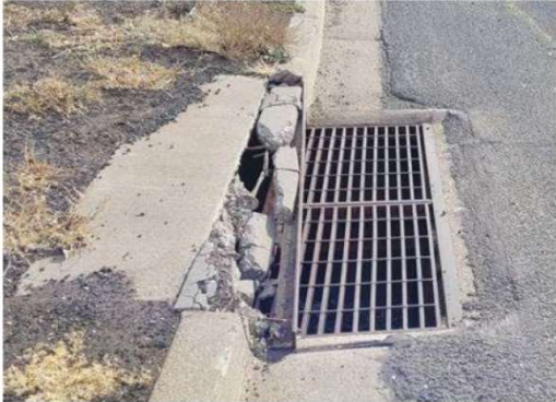
Figure 2 – Damaged catch basin view 1
