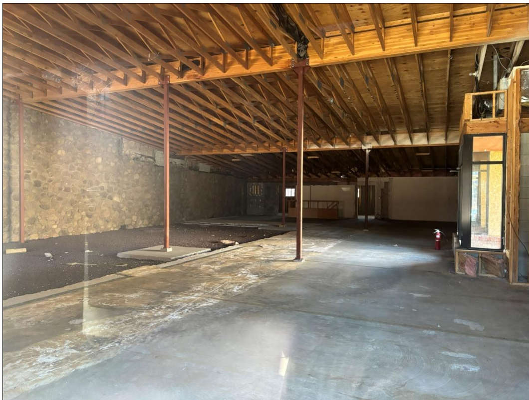
Photograph 5. The interior of 111 N Leroux Street, looking west, the original 1949 construction is located along the cinder area to the left. The southern wall of the building appears to be original and is shared with the neighboring building.
