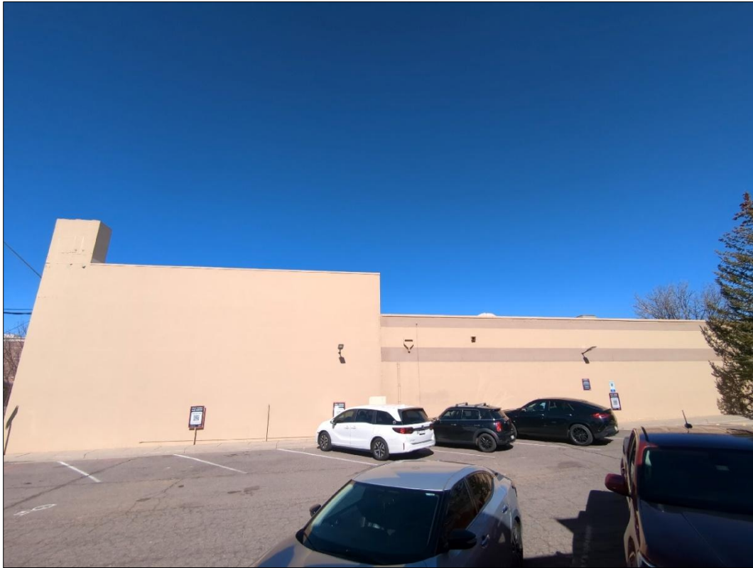
Photograph 2. North facing view of 123 North Leroux showing the southern face of the building and the parking lot adjacent to the building to the south.
