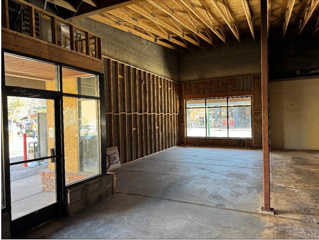
Photograph 6. The interior of 111 N Leroux Street, looking east out to Leroux Street, the original 1949 construction begins roughly at the beam and proceeds south, east, and west. All the interior of the building has been gutted, displaying structural elements.
