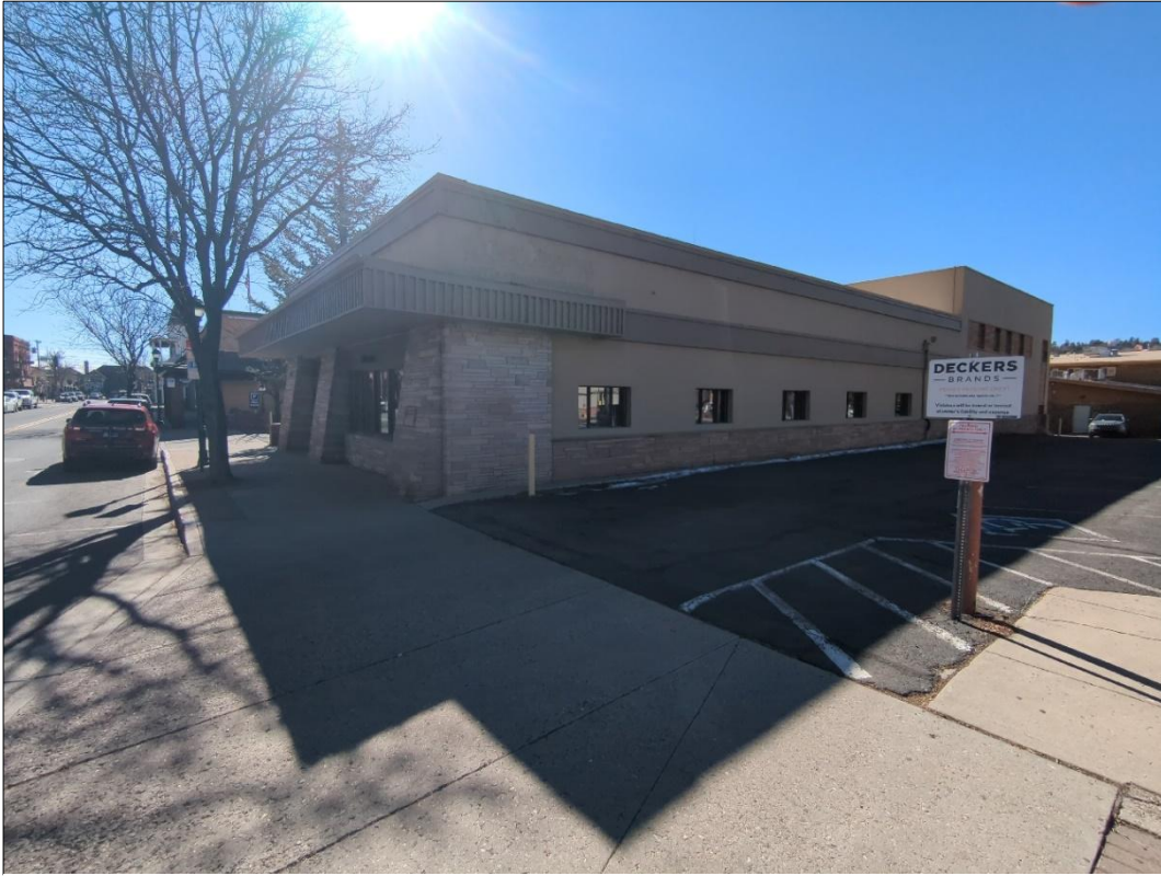
Photograph 3. Southwest facing view of 123 North Leroux showing the northern and western faces of the building. The sandstone footers, vinyl canopy, and sandstone piers are visible in the photograph.
