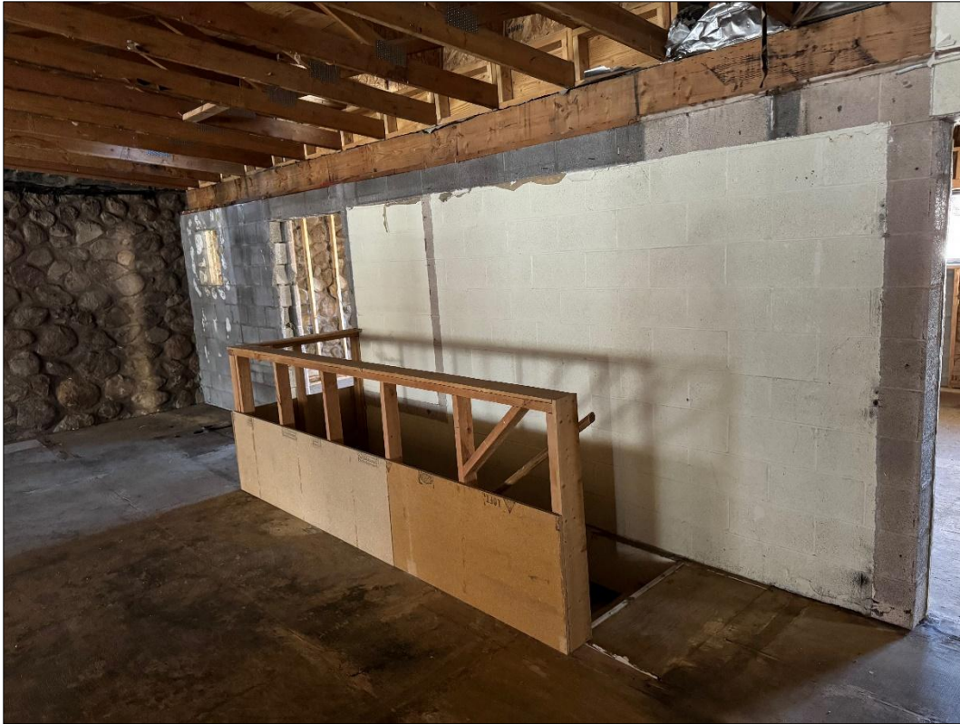
Photograph 4. The interior of 111 N Leroux Street, looking southwest, the access to the original 1949 basement is in the forefront of the image, while the westernmost section of the 1994 addition begins at the cinderblock wall behind the stairway. The malpais southern wall is original and is shared with the neighboring building.
