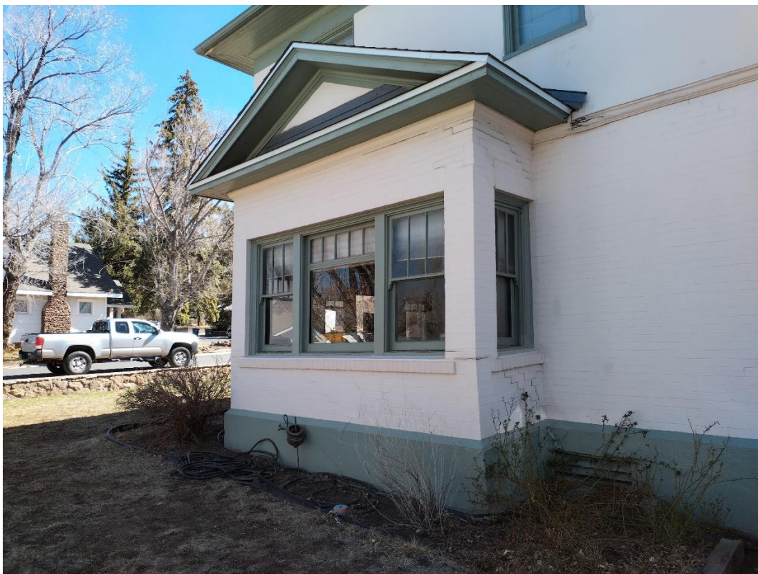
Photograph 7: West elevation bay projection needing reconstruction
