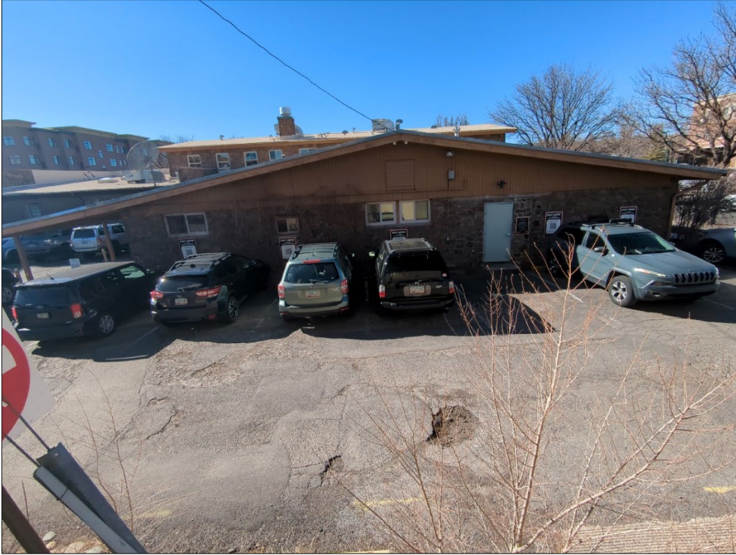
Photograph 6. East elevation of 19 W Birch Ave, showing the east facade of the former police station.
