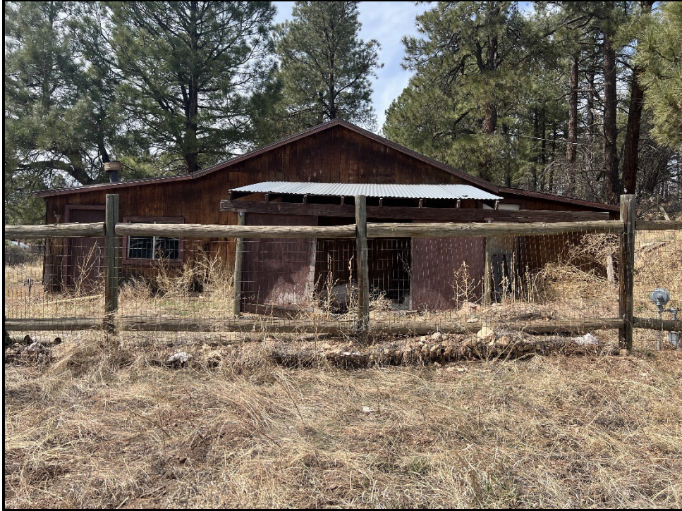
Figure A-9. East elevation (entrance) of Unit 2, street view from South Lake Mary Road; view facing west.
