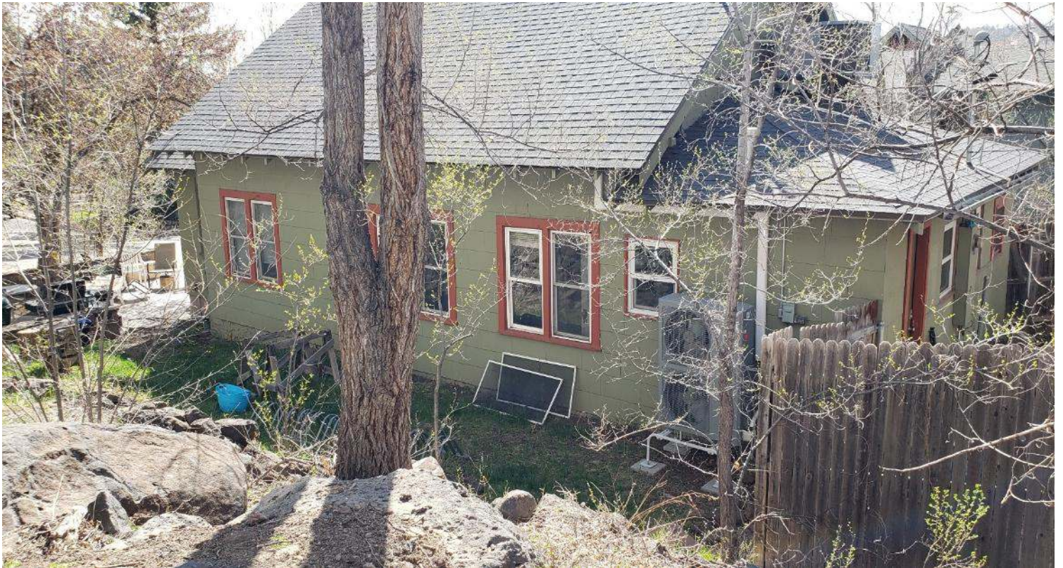
Photos 15–16. 418 E Birch Ave rear/NNE façade facing SSW (top) and E façade & rear facing W (bottom).
