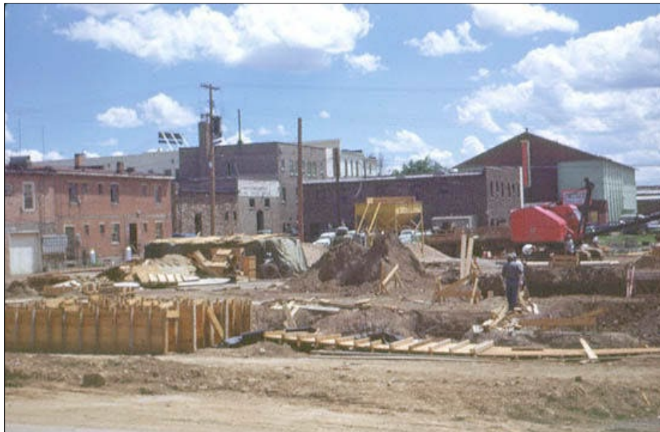
Photograph 2. Photograph of the initial stages of construction of City Hall in 1951 (Babbit 1950).
