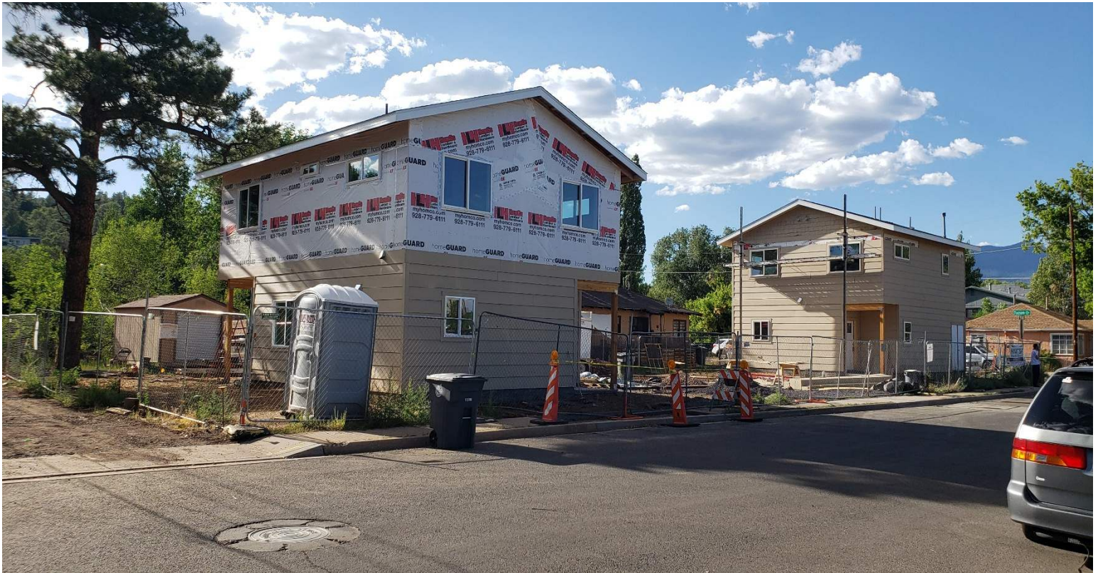
Photos 5–6. 205 S Park St interior wall showing modern dimensional lumber and sheetrock where ca. 2015 plumbing repair was made (top) and 205 S Park St location to NW showing new house construction with 407 W Tucson in background between two new structures and 407 W Tucson outbuilding in left background (bottom, also 123 S Park St house in far-right background).
