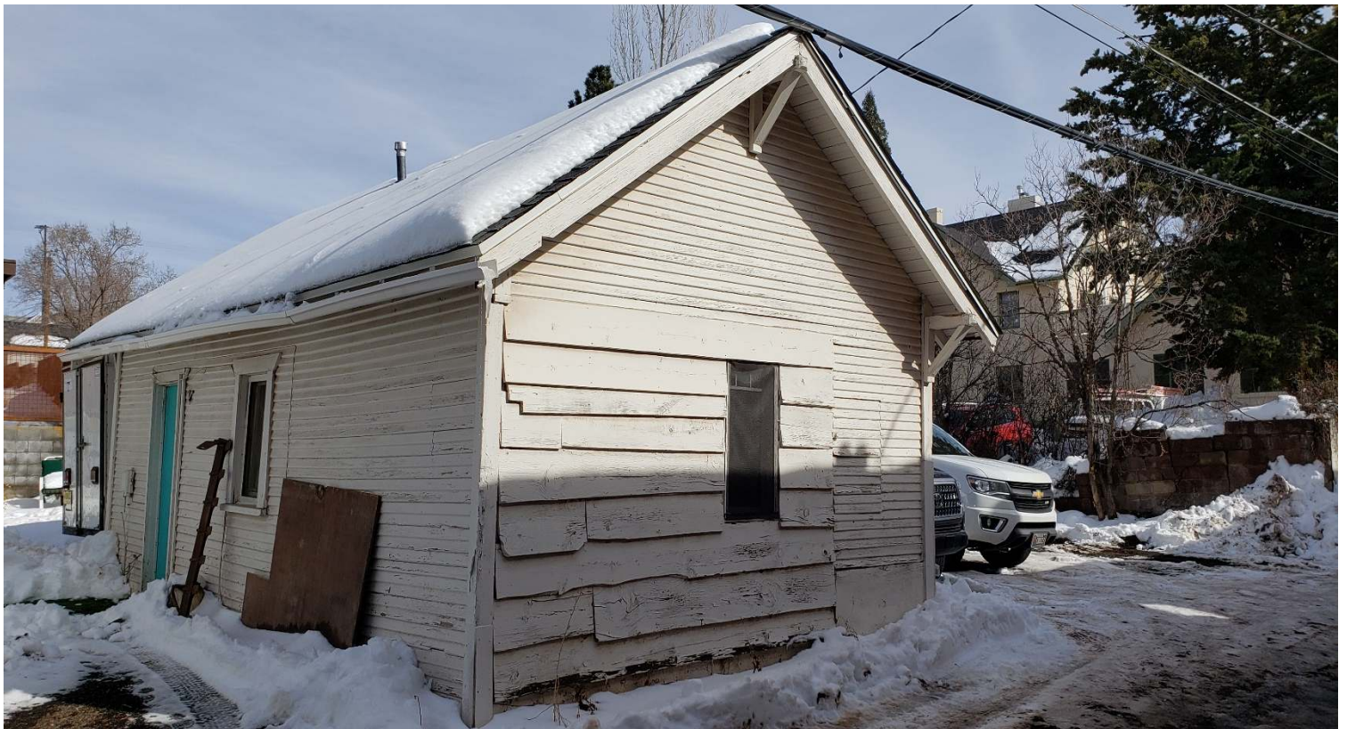
Photos 3–4. 314 N Beaver St house SE corner, Unit 4 (with blue door), Unit 5 (left of Unit 4) overview to NE (top) and Unit 4 S and W façades facing NE (bottom).
