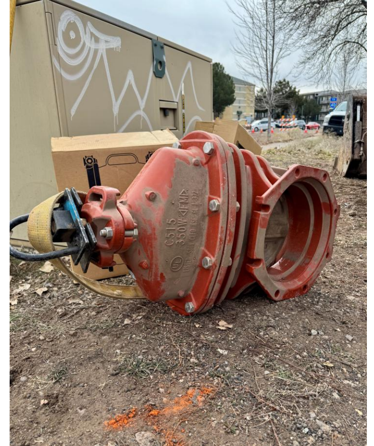
Wednesday: Valve waiting to be installed restores water to affected customers while also isolating the break location for repair.
