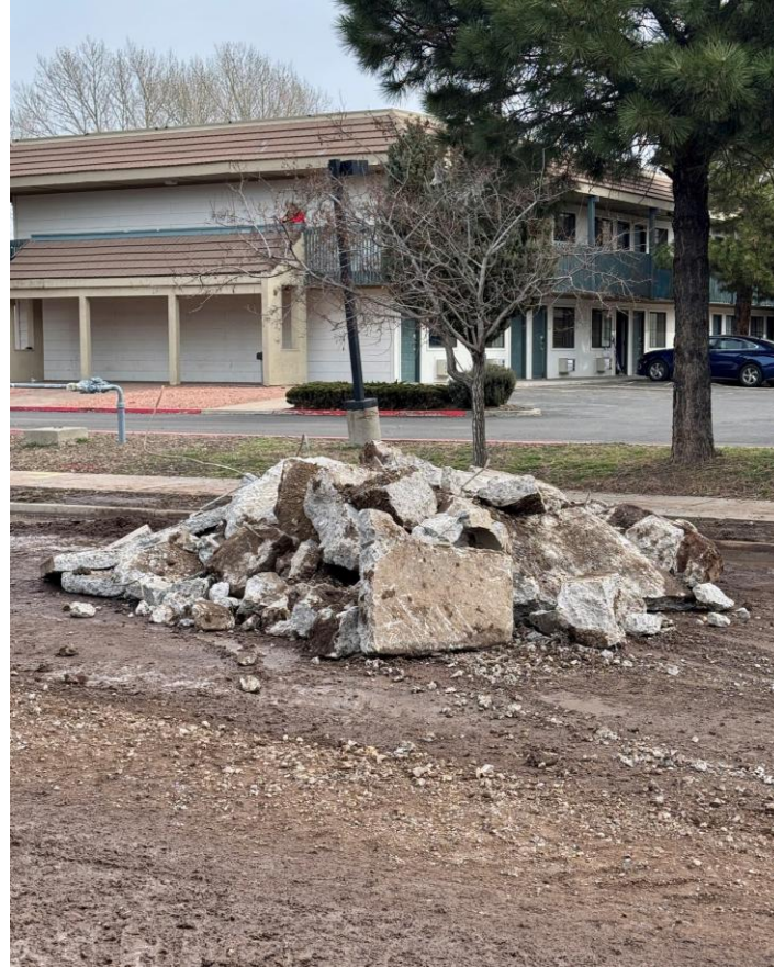
Wednesday: Debris of the stormwater collection basin that had to be removed before water main could be repaired.
