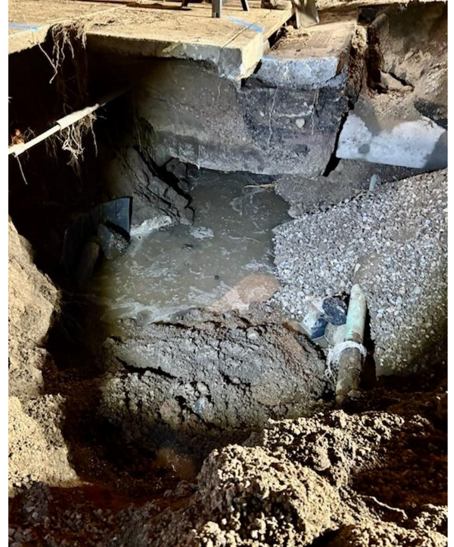
Photo of water main break taken at 1:15 a.m. Wednesday morning.
