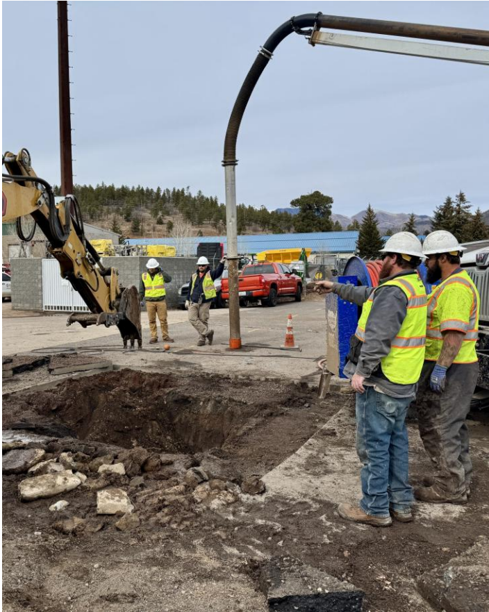
Wednesday: City Water Services crews prepare a 2 nd site to install valve that returns flow to remaining properties.
