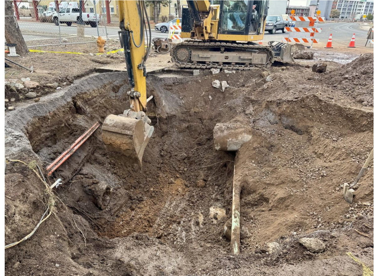
Wednesday: Site of main break shows proximity of utilities to water main, including natural gas directly above and to the right, and fiber optics and irrigation above and to the left.
