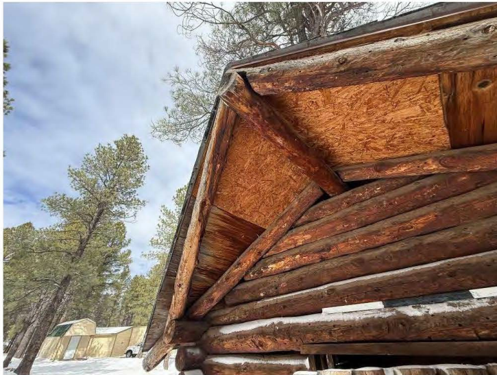
North wall roof details of Small Cabin, view northwest, scale is 3 feet.
