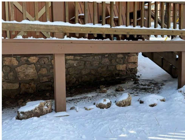
North wall and deck and foundation details of Cabin Ten, view south.
