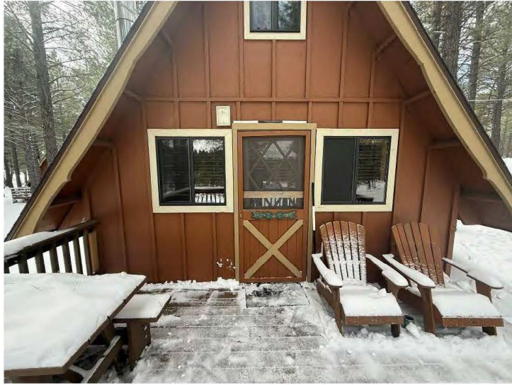
North wall, door and deck of Cabin Six, view south, scale is 3 feet.
