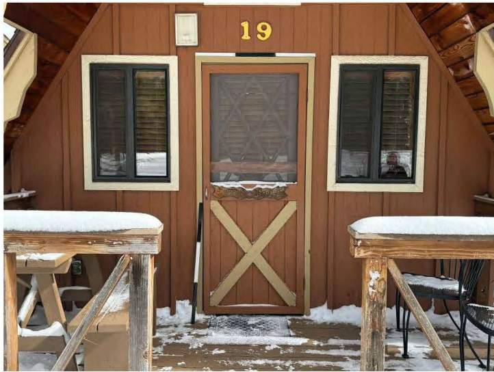
South wall, window and door details of Cabin Nineteen, view north, scale is 3 feet.
