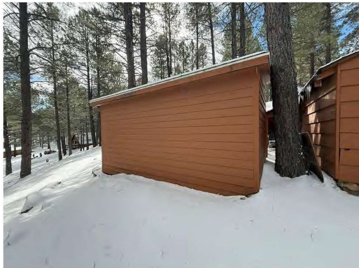
North wall of shed adjacent to east of Cabin Sixteen, view south.
