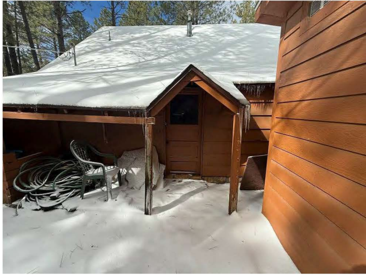
East entrance and open sheds on east wall of Cabin Sixteen, view west.
