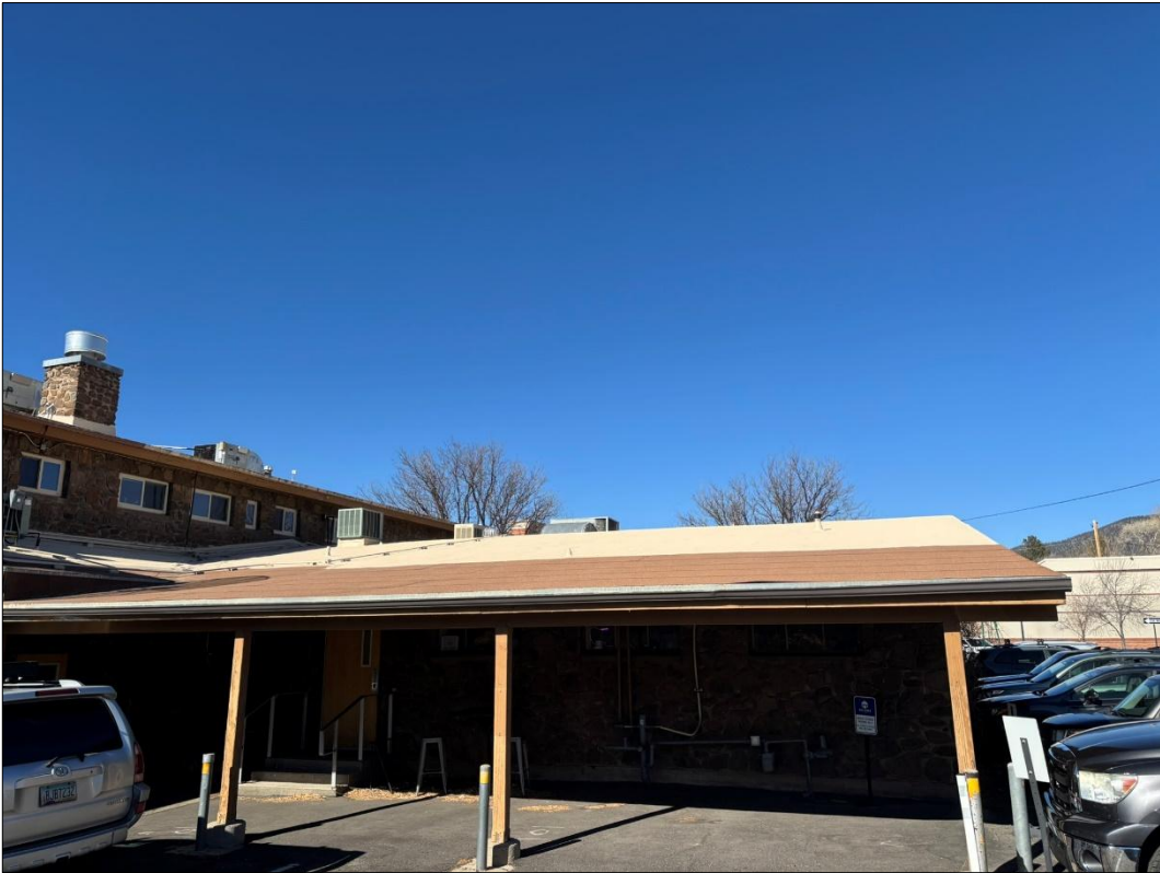
Photograph 8. South facing facade of the former fire department, showing the extension of the roof which forms a canopy.
