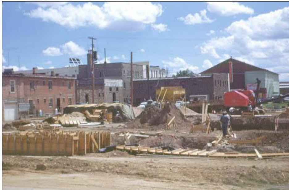
Photograph 2. Photograph of the initial stages of construction of City Hall in 1951 (Babbitt 1950).
