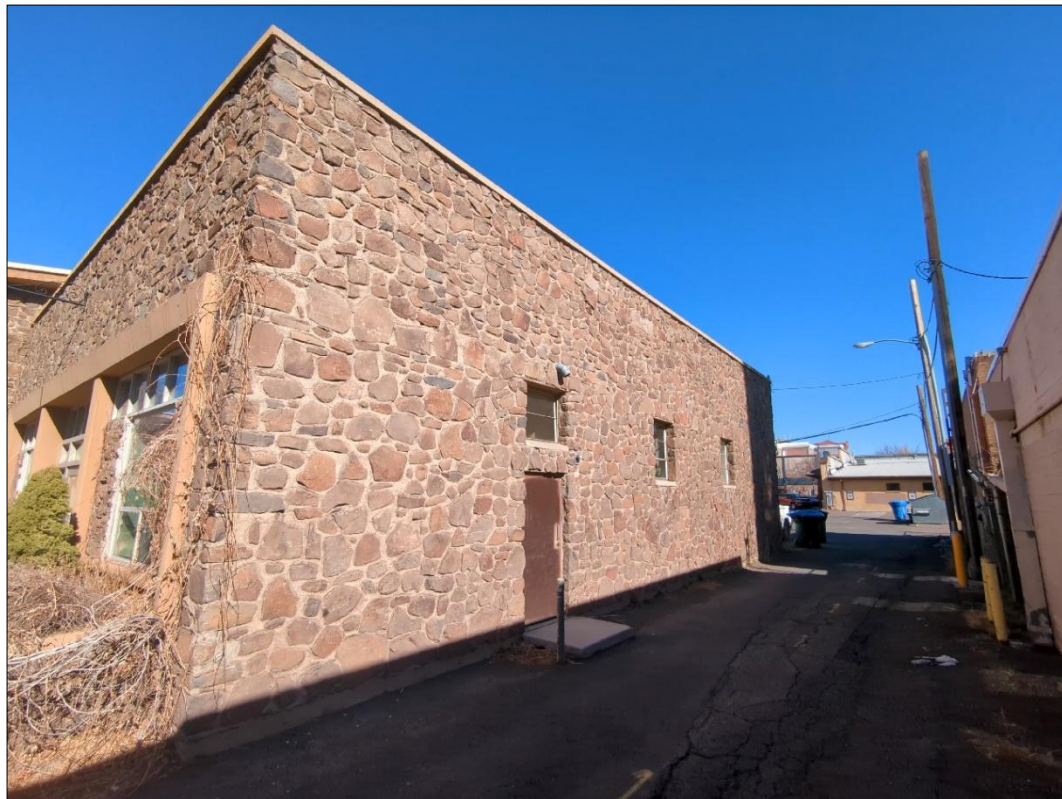
Photograph 6. South facing exterior of the former fire department, which exits into an alleyway.
