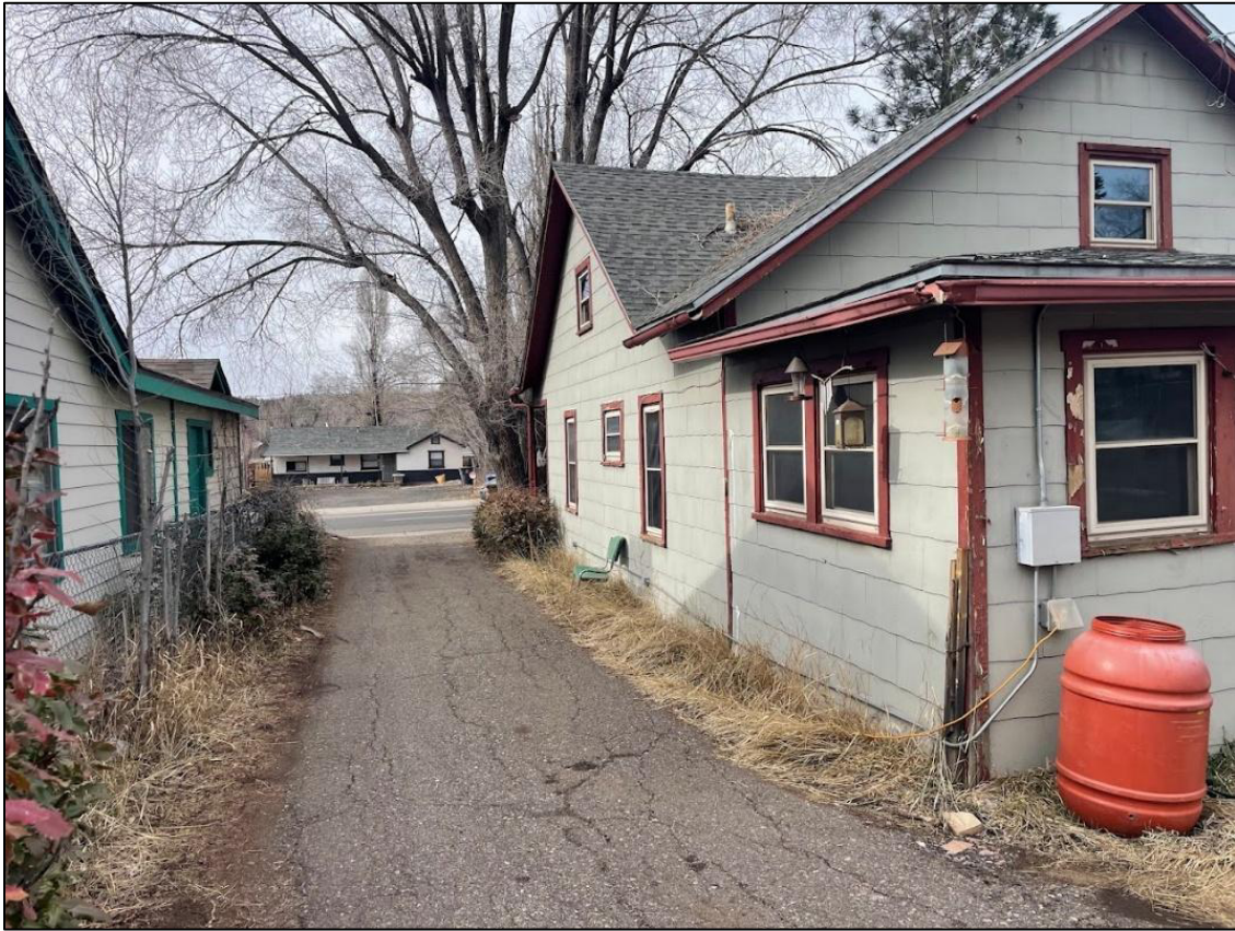
Photograph 8. West elevation showing settlement at porch
