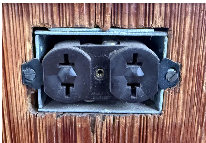
Photograph 7. Representative overview of an ungrounded electrical outlet at 804 ½ North LeRoux Street, facing north.
