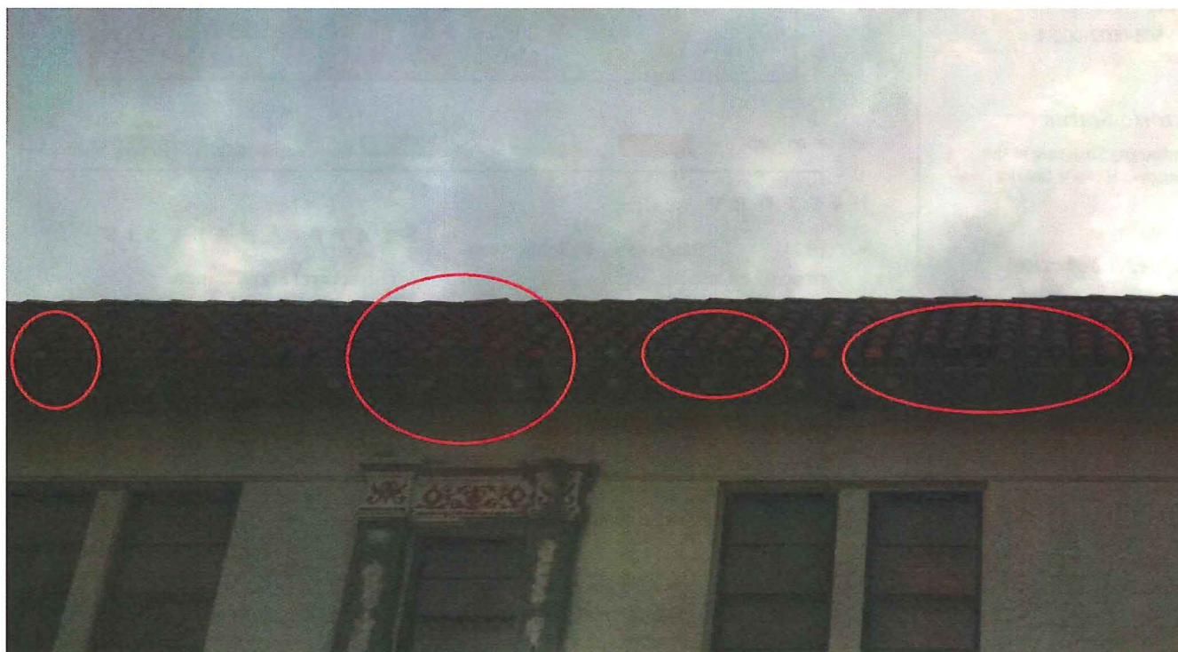
Photo of the existing conditions revealing damaged tiles
