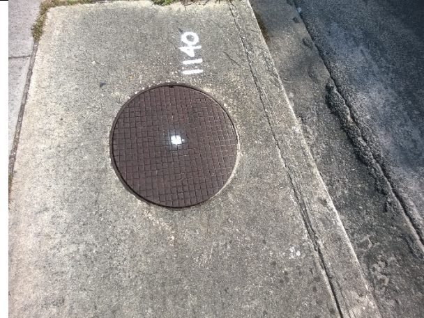
Photo 14: View of stormwater drain located in east side of site along N 17 th Street.
