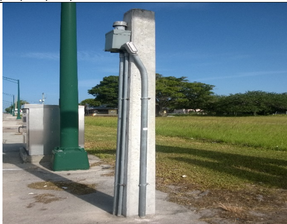
Photo 11: View of traffic signal control in southeast corner of site.
