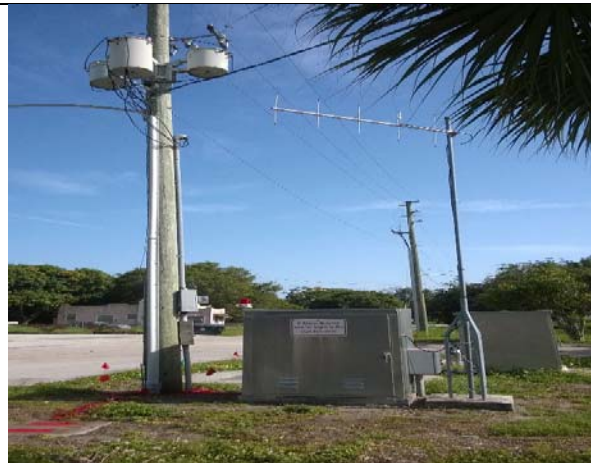
Photo 15: View of pole-mounted electrical transformers and lift station in southwest corner of site.
