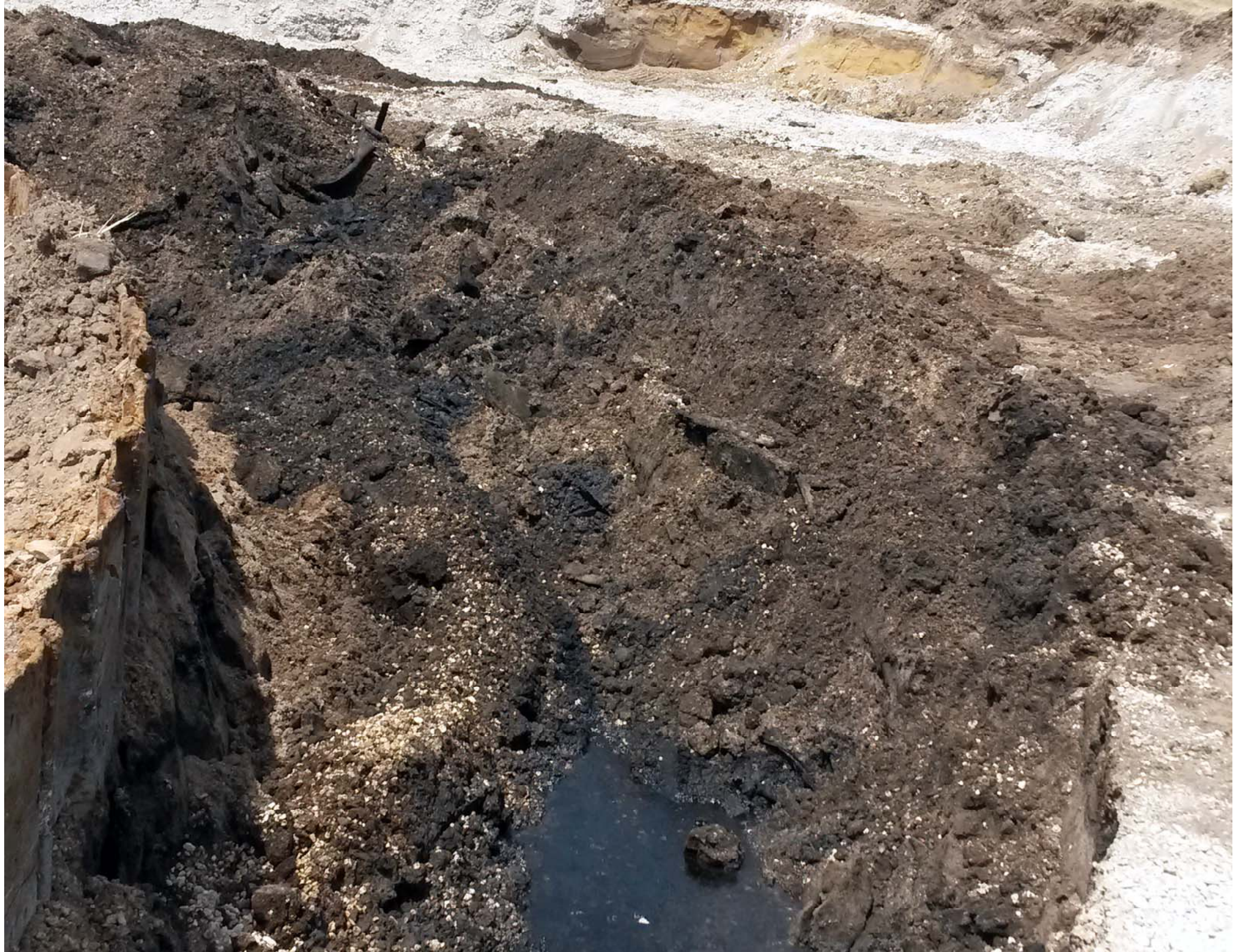
King Plant Property - Contaminated material below design depth - April 7, 2014
