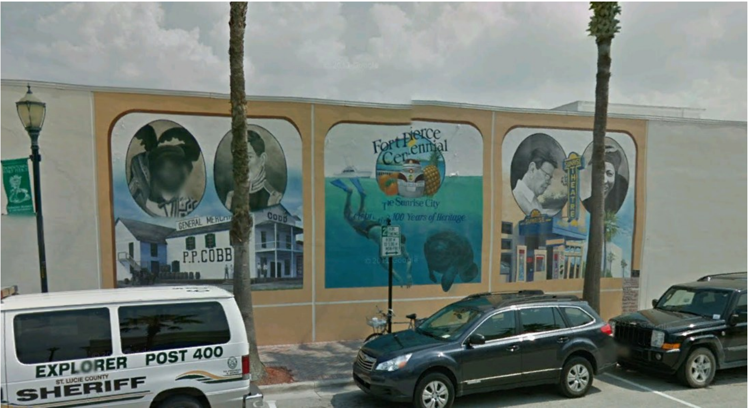
Avenue A, Between N 2nd St. & N Indian River Dr. Mural on Former OPS Building— Currently deteriorating
