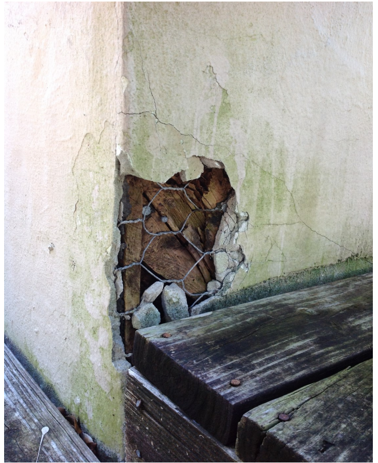
Structural & Stucco Damage as indicated by the Representative
