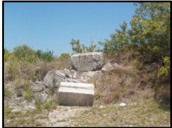
PHOTOGRAPH #04: CONCRETE RUBBLE LEFT ON-SITE
