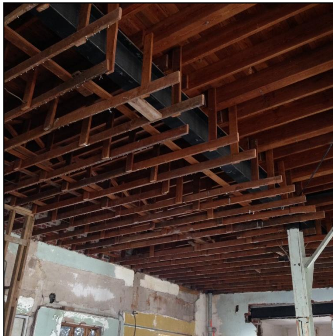
Exposed interior walls and ceilings
