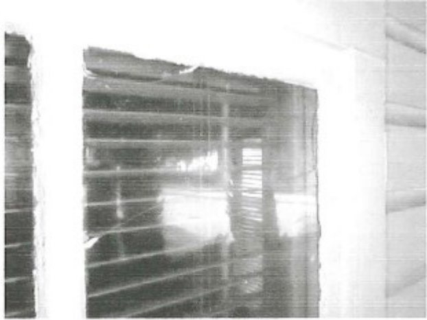
Broken Glass Top Panes are fixed in place existing double hung does not work
