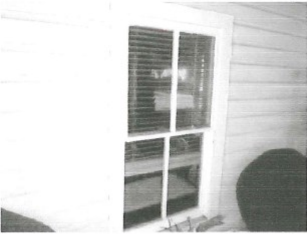
Original Window Design to be replaced with replica Double Hung with split design
