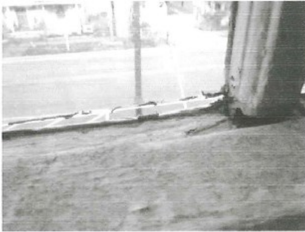
Rotted Sills with gaps Not able to repair again
