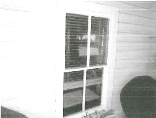
Original Window Design to be replaced with replica Double Hung with split design
