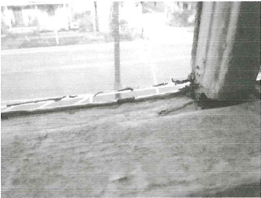
Rotted Sills with gaps Not able to repair again
