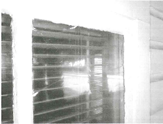
Broken Glass Top Panes are fixed in place existing double hung does not work
