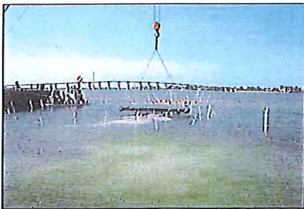
PVC stakes were used as guides for the mattress placement. A crane roughly placed the mattresses, and divers made the final adjustments.
