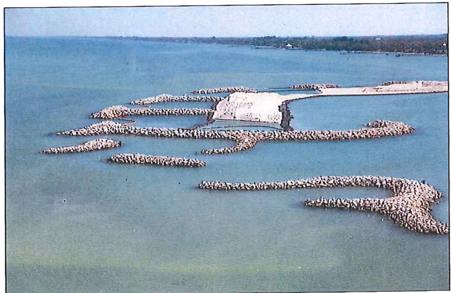
This shows the islands construction progress on March 15. The marina project will soon go out to bid, expecting to begin construction in July. (Photos by Steve Irwin of Island Marine Electronics)
