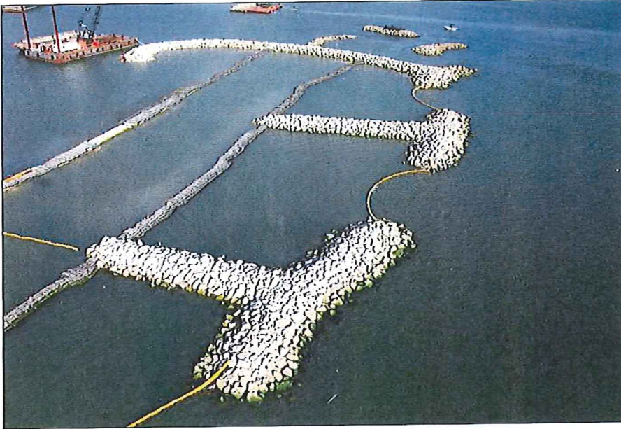
In December 2012, the contractor continues building the man-made storm protection islands for the city marina in Fort Pierce, Fla. (Photos by Steve Irwin of Island Marine Electronics)
