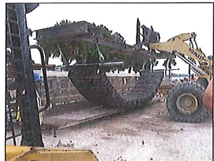
The 12-inch mats required a filling frame, fabricated by the contractor. The panels came pre-assembled with the exception on the side panel, through which a front-end loader placed the stone fill. Then, the side panel was attached and loaded into the stockpile.
