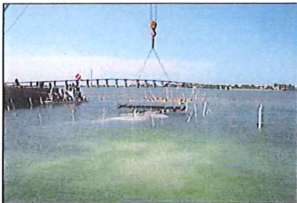
PVC stakes were used as guides for the mattress placement. A crane roughly placed the mattresses, and divers made the final adjustments.
