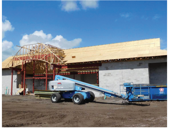
Trusses and roof sheathing being installed at Cumberland Farms on 35 th St.
