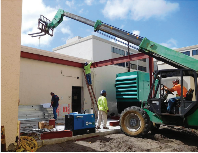
Steel beams being erected for the angiography suite during the Lawnwood Hospital renovation.
