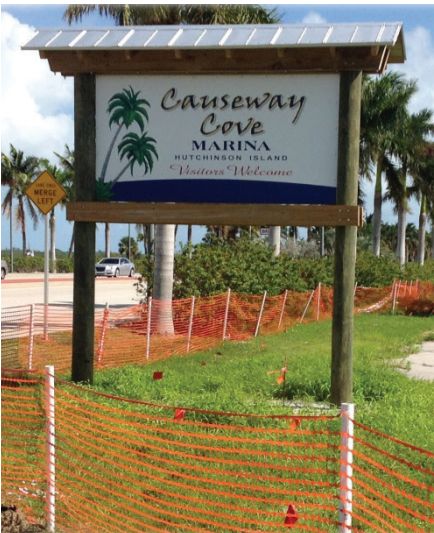
Construction of Causeway Cove Marina is underway to establish a 198 slip marina, boat ramp, dock master's quarters, ship store, and 10 recreational vehicle (RV) spaces at 601 Seaway Drive.
