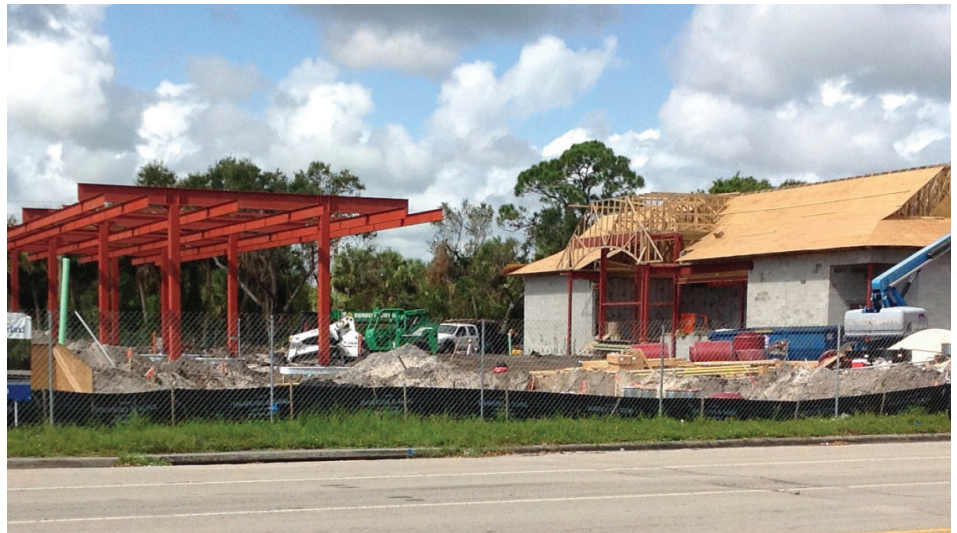
Construction of the new Cumberland Farms, Inc has begun adjacent to Indian River State College at 2009 S. 35th Street. This 4,900 sq. ft. store will provide 16 service pumps within a Florida Vernacular theme.
