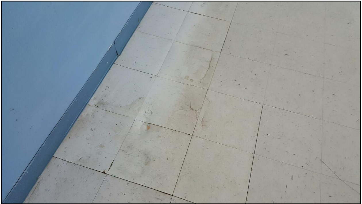
VIEW OF FLOOR DAMAGE IN ONE OF THE CLASSROOM AREAS
