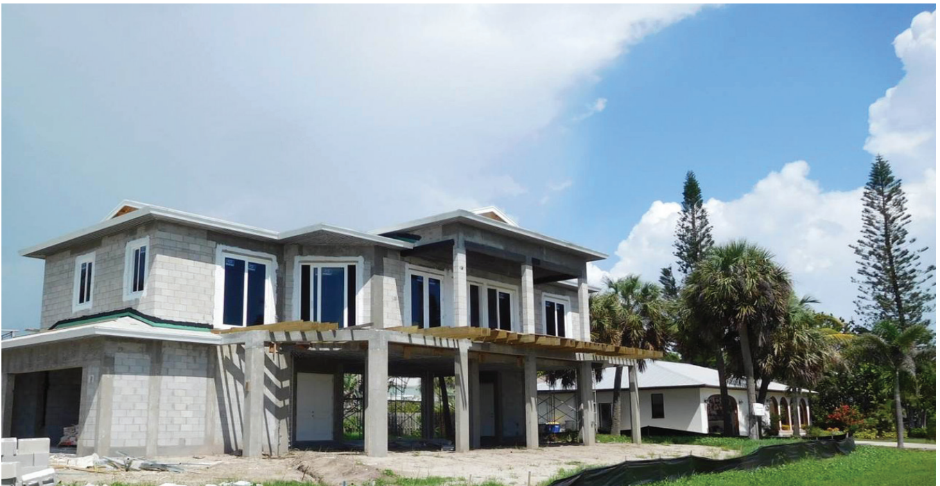
1709 Surfside Drive- The single family home shown above is located in a special flood hazard area. In addition to complying with Florida Building Code requirements, the elevation of the structure is consistent with the approved construction methods according to Paul Thomas, Building Official and Certified Floodplain Manager. This picture was taken during the drywall inspection; the next inspection scheduled is for stucco which will be completed shortly.
