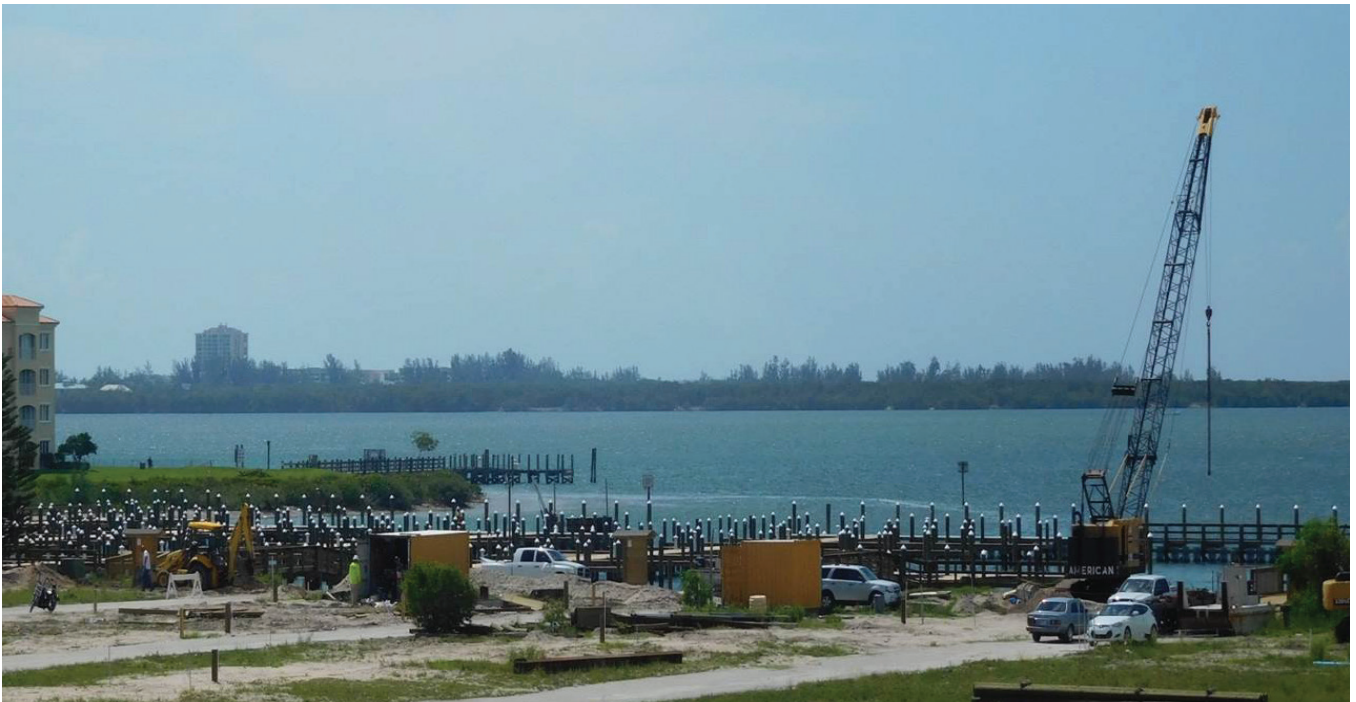
601 Seaway Drive, Causeway Cove Marina- This photo shows the 8 docks that completed first electrical and plumbing inspections. The next step will be the installation of the fire department connections. .....
