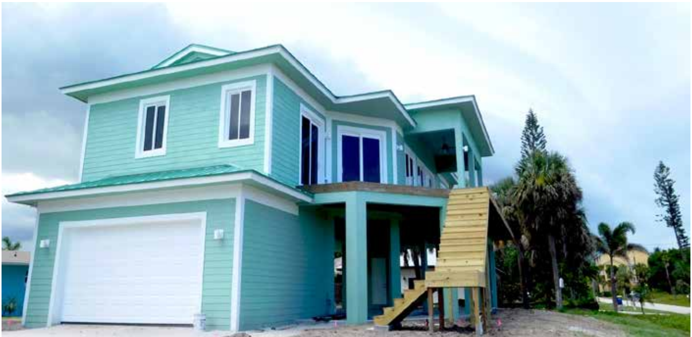
1709 Surfside Drive- This home is nearing completion with only final inspections remaining. This photo was taken while Inspector Granadillo inspected the A/C system. This house exemplifies the approved construction techniques required in the flood zone. The garage is constructed of engineered “breakaway walls,” designed to break away in flood conditions to prevent/minimize damage to the rest of the structure.
