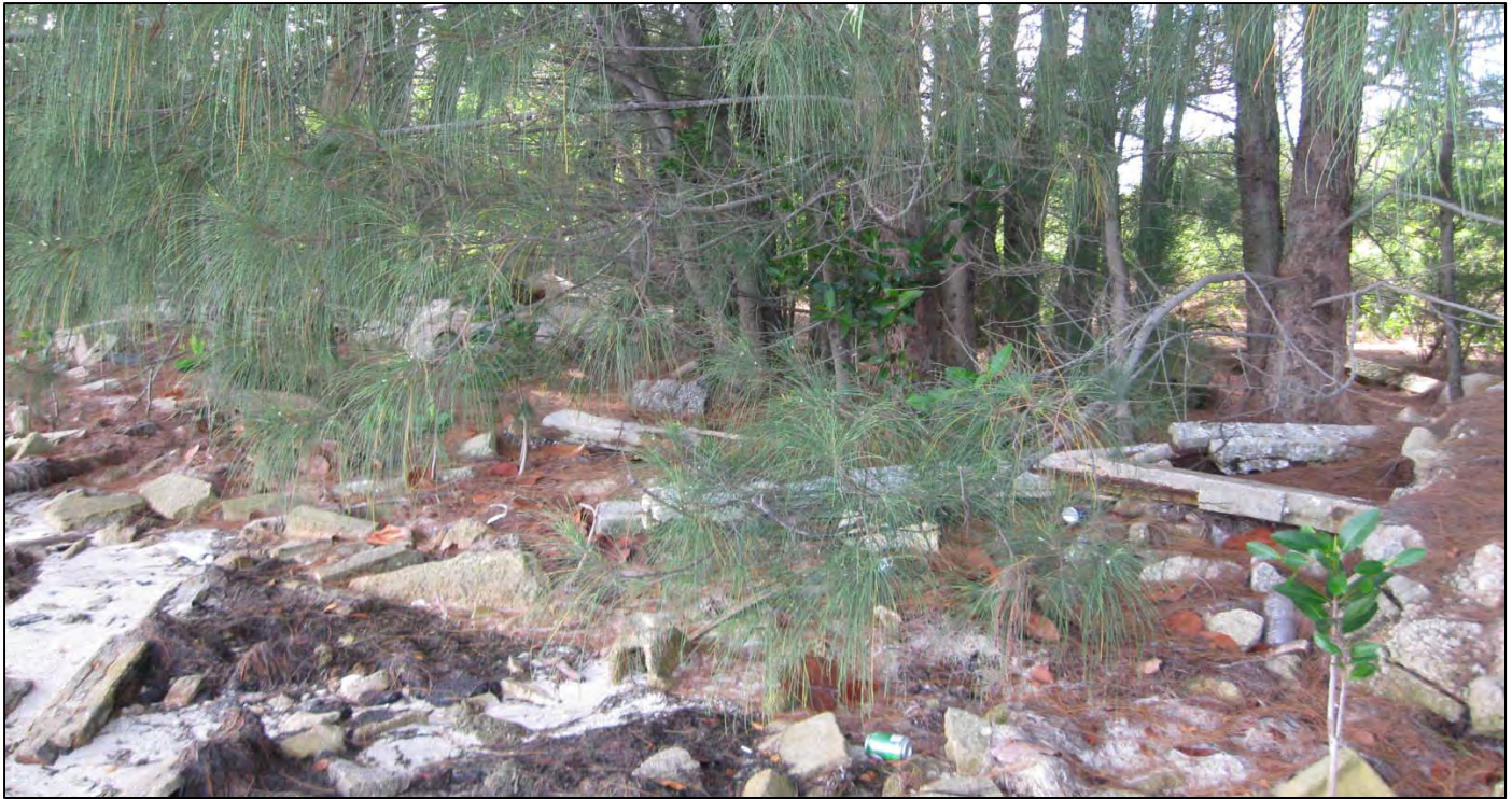
Photo looking at concrete rubble in shoreline area.
