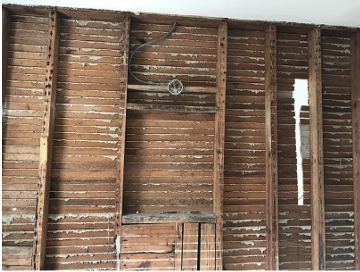
Damaged elements – pictures provided by the applicant
