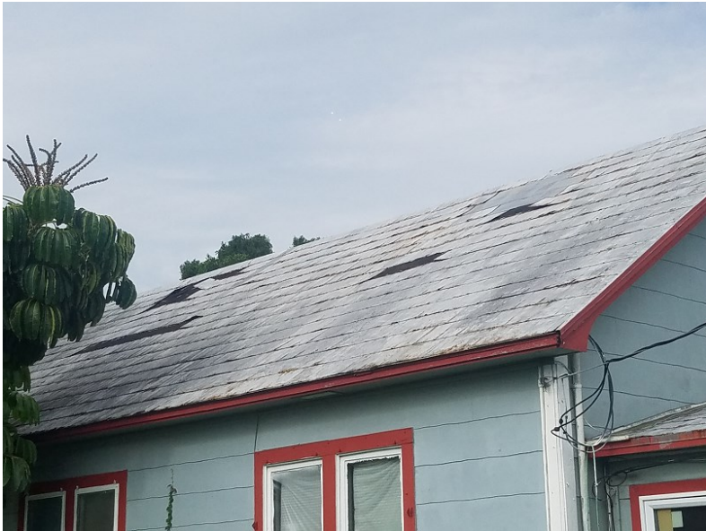
East side roof to be replaced
