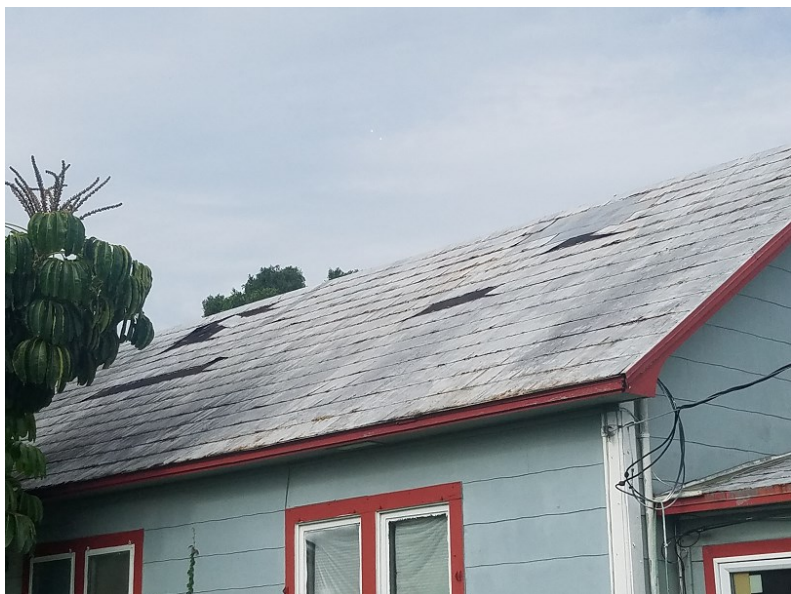
East side roof to be replaced
