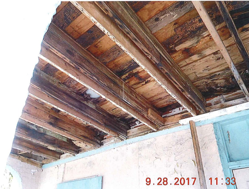
Damaged elements — pictures provided by the building inspector
