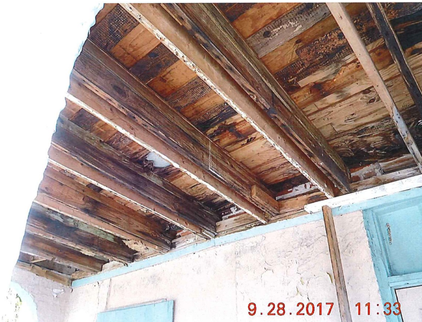
Damaged elements — pictures provided by the building inspector
