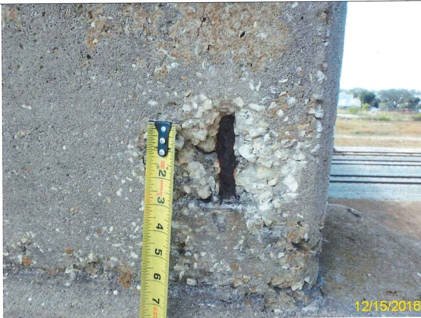
Photo 9 - Element 321 Re Conc Approach Slab
