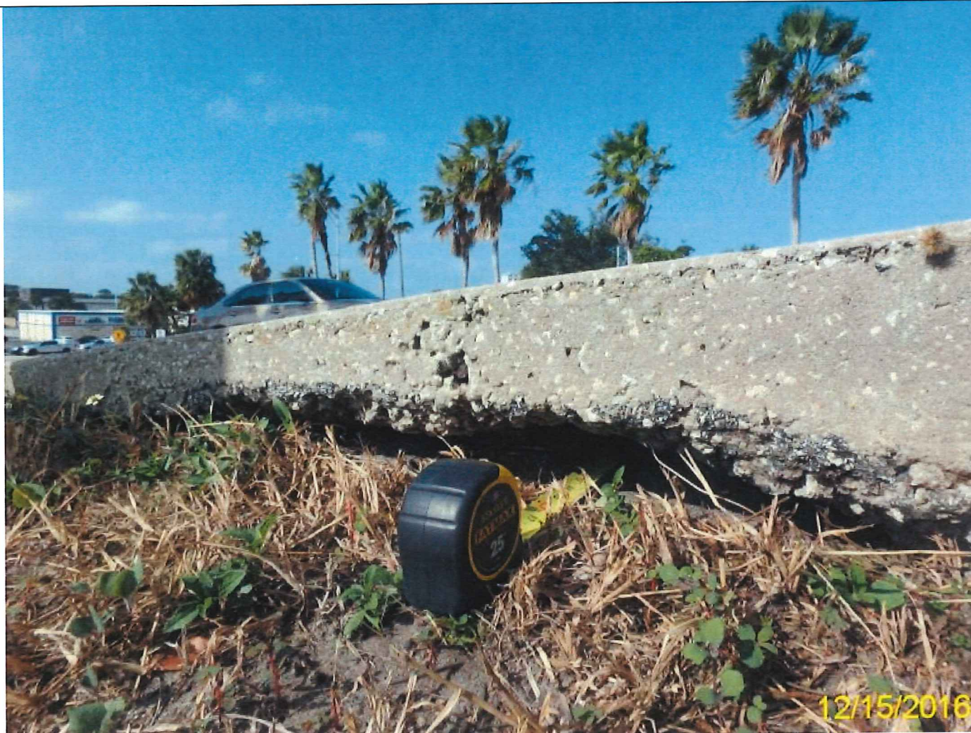
Photo 8 - Element 321 Re Conc Approach Slab
