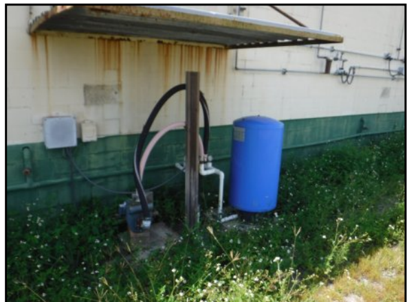
48 : Previous potable water well
