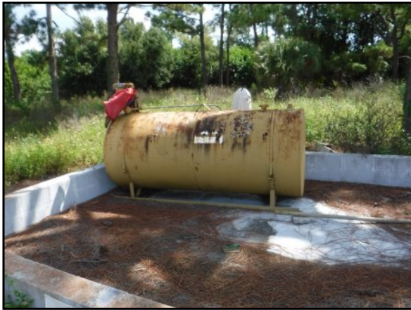
33 : Diesel fuel AST in secondary containment
