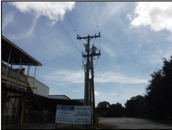
67 : Pole mounted transformers along southern adjoining street
