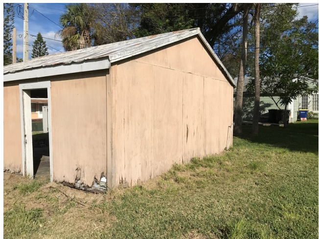
Pictures showing extensive deterioration of the structure.
